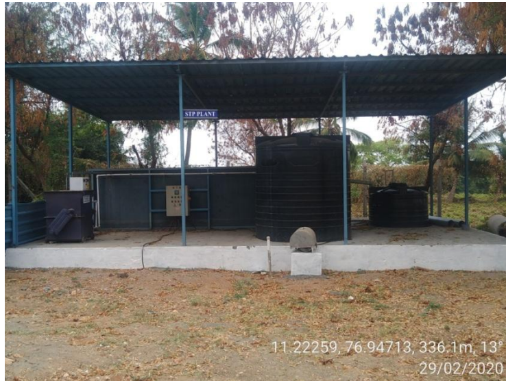
Sewage Treatment Plant
