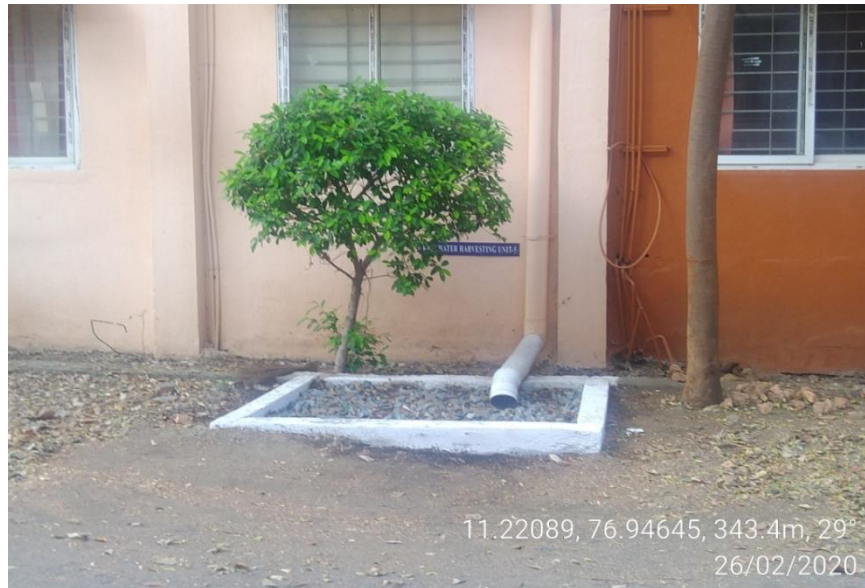
Rain Water Harvesting Units
