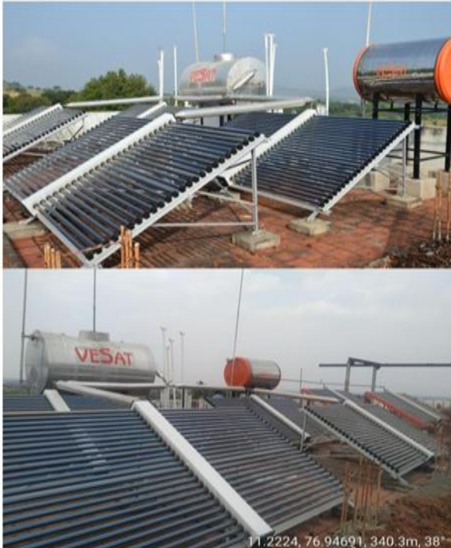
Solar Water Heater at Boy's Hostel
