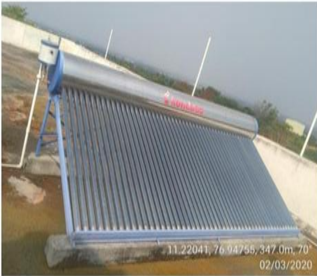
Solar Water Heater at Girl's Hostel
